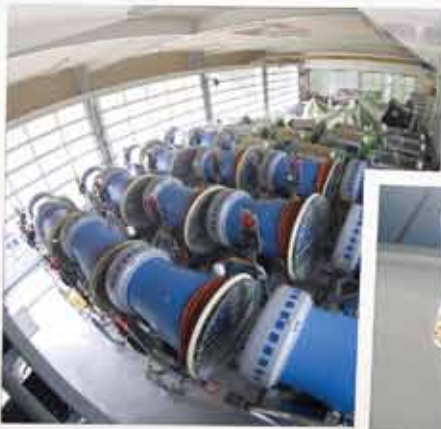
Snow cannon storehouse K1 Schlegelkopf (= compressor station)
